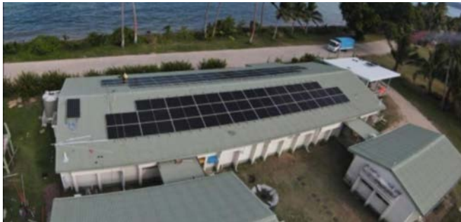
Solar installation - Lomaloma, Vanua Balavu, Lau
