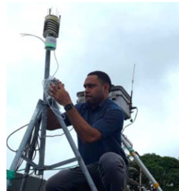
Installation of air quality devices
